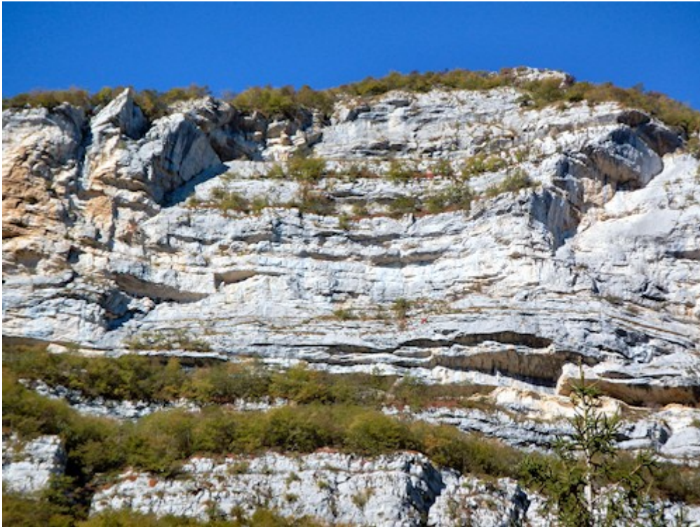
The horrible slope to the East of Monte Cornale between Lake Garda and Adige valley
